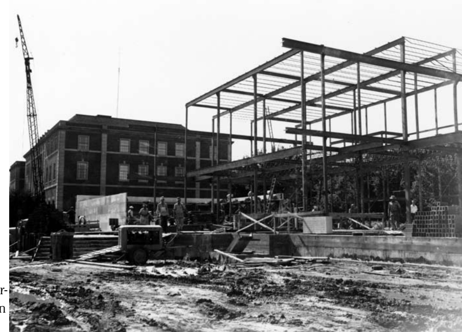
Construction of the NSHS Headquarters building, July 25, 1952. We selected this photo because you can see the foundation. NSHS RG14-7-3
