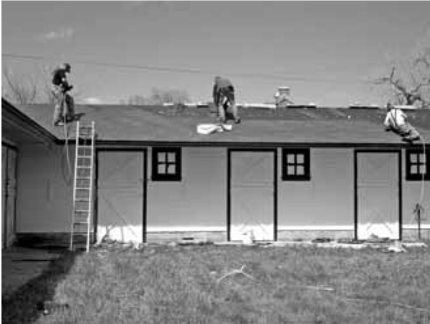
Maintenance crew re-shingles the Veterinary Hospital annex in April 2005: Left to right, Charley McWilliams, Steve Scoggan, Bryce Darling. Photo by Curt Peacock
