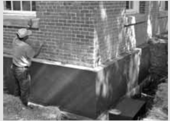
Charley McWilliams tuck-points a mortar bond between bricks. Photo by Curt Peacock
